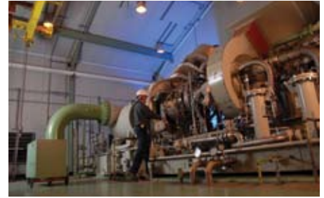
Operator personnel monitoring turbine engine performance.
