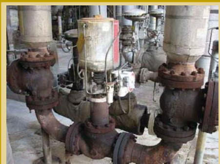
Uninsulated piping near control valve
