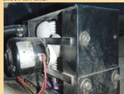
No guard protection for fan blades
